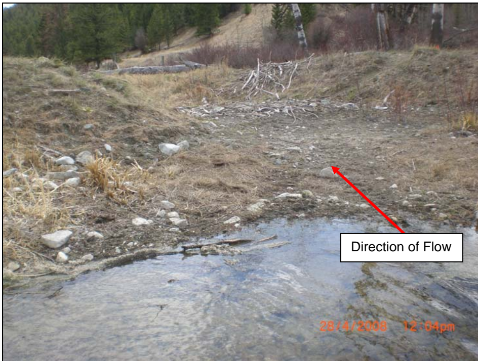
PHOTO A8 – JACLAKE Dry Spillway
